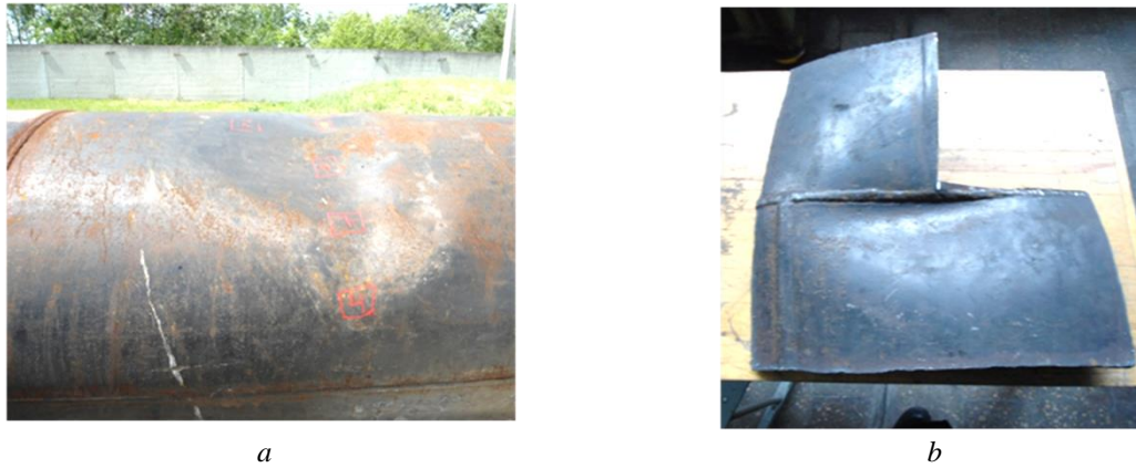
Figure 4. The plastic deformation areas of pipeline detected using the inside-pipeline diagnostics: a – deformation of pipe body; b – deformation of metal in the areas of weld seams
