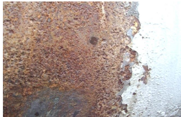
Figure 3. Corroding defects detected using the inside-pipeline diagnostics
